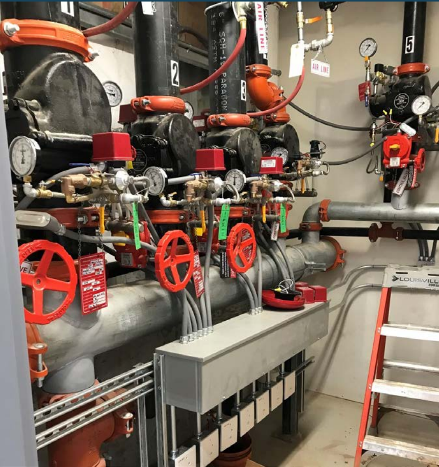
Sprinkler Riser Room
