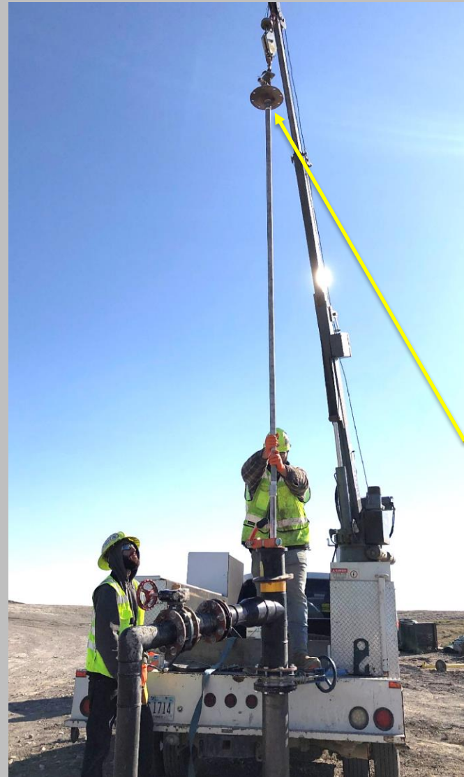
Strap and hoist the final hard pipe with top-head steel-flanged wellhead, discharge tee and landing plate attached
