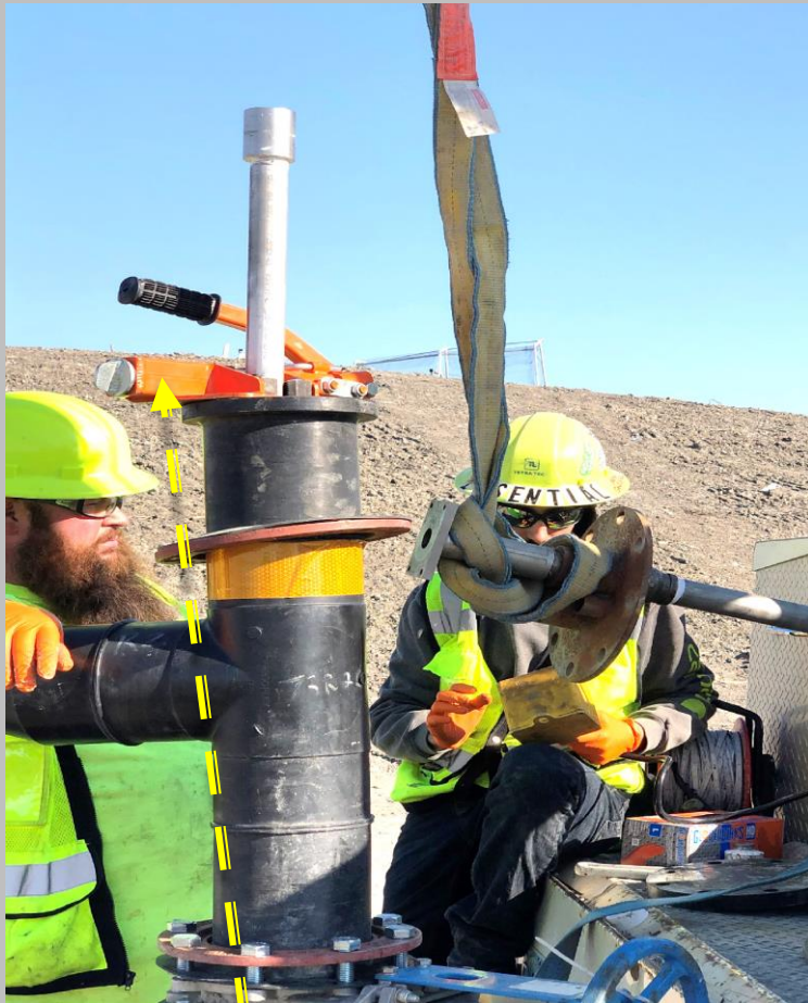
Orange top-head clamp with drain coupling on flanged wellhead casing
