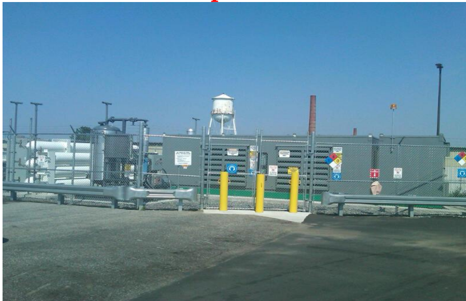
Natural Gas Delivery & Compression
